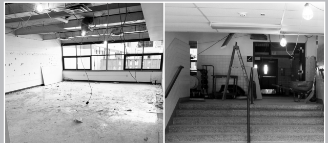
Flooring, cabinets and ceilings have been removed from classrooms at Chenango Bridge.
